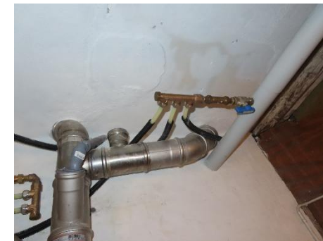
Messingfitting i rustfri installation
