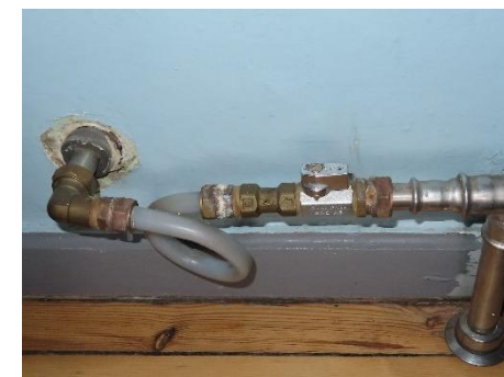
Messingfitting i rustfri installation
